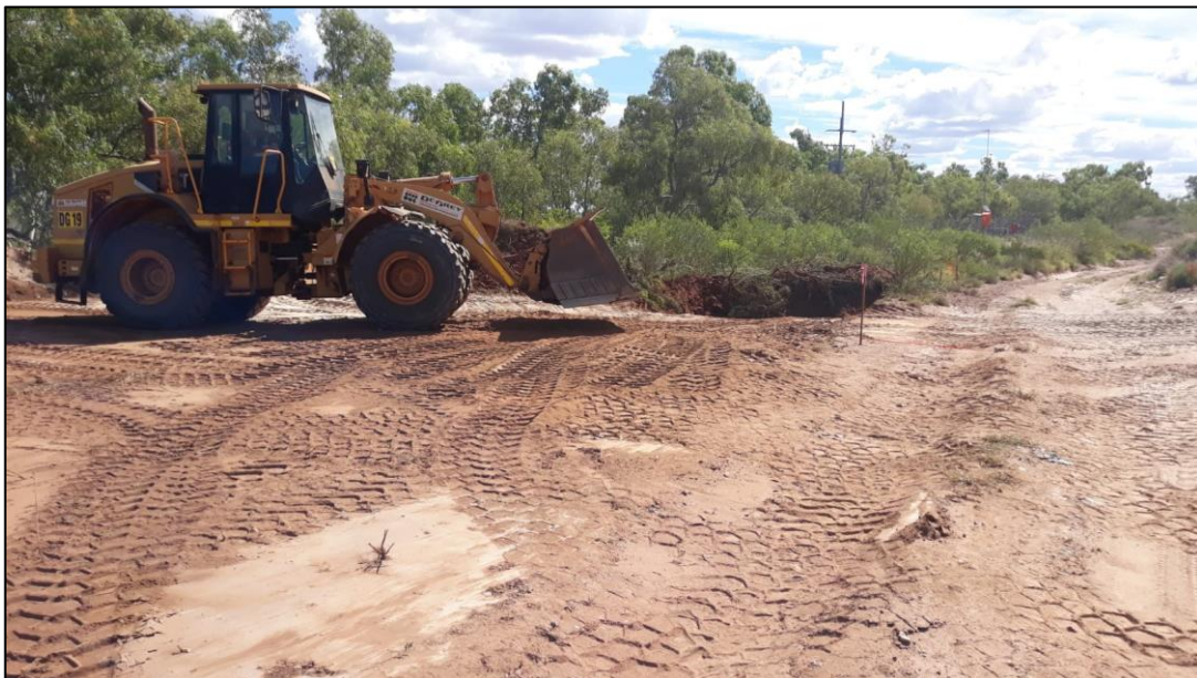
Figure 1: Loader preparing drill pads for the upcoming drilling program at the Mt York Project.
