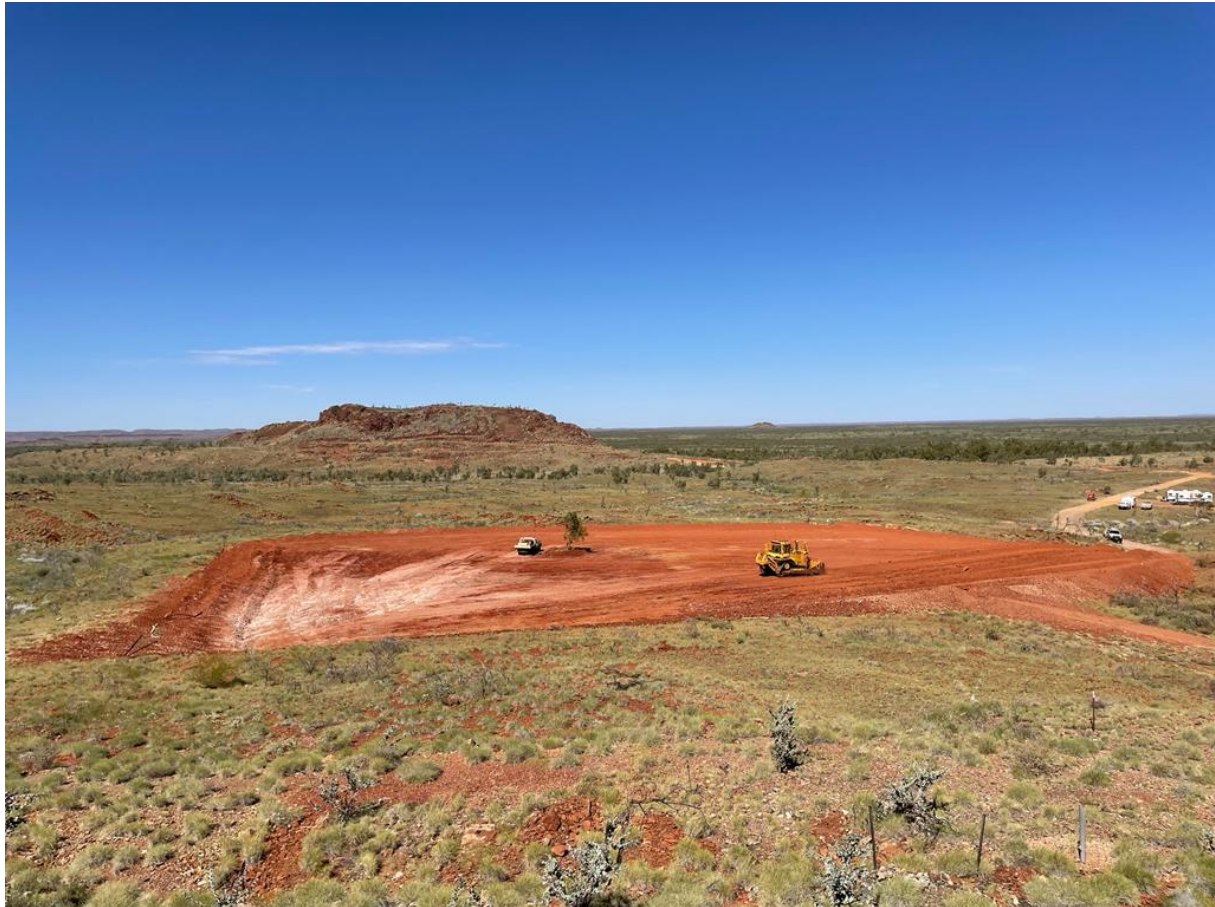
Figure 15. Exploration camp construction underway with levelling and compaction of 70m x 70m area in preparation for dome-sheltered core yard, accommodation, ablution block, workshop and offices. The prominent hill in the background is the part of the Main Hill prospect. View looking south.
