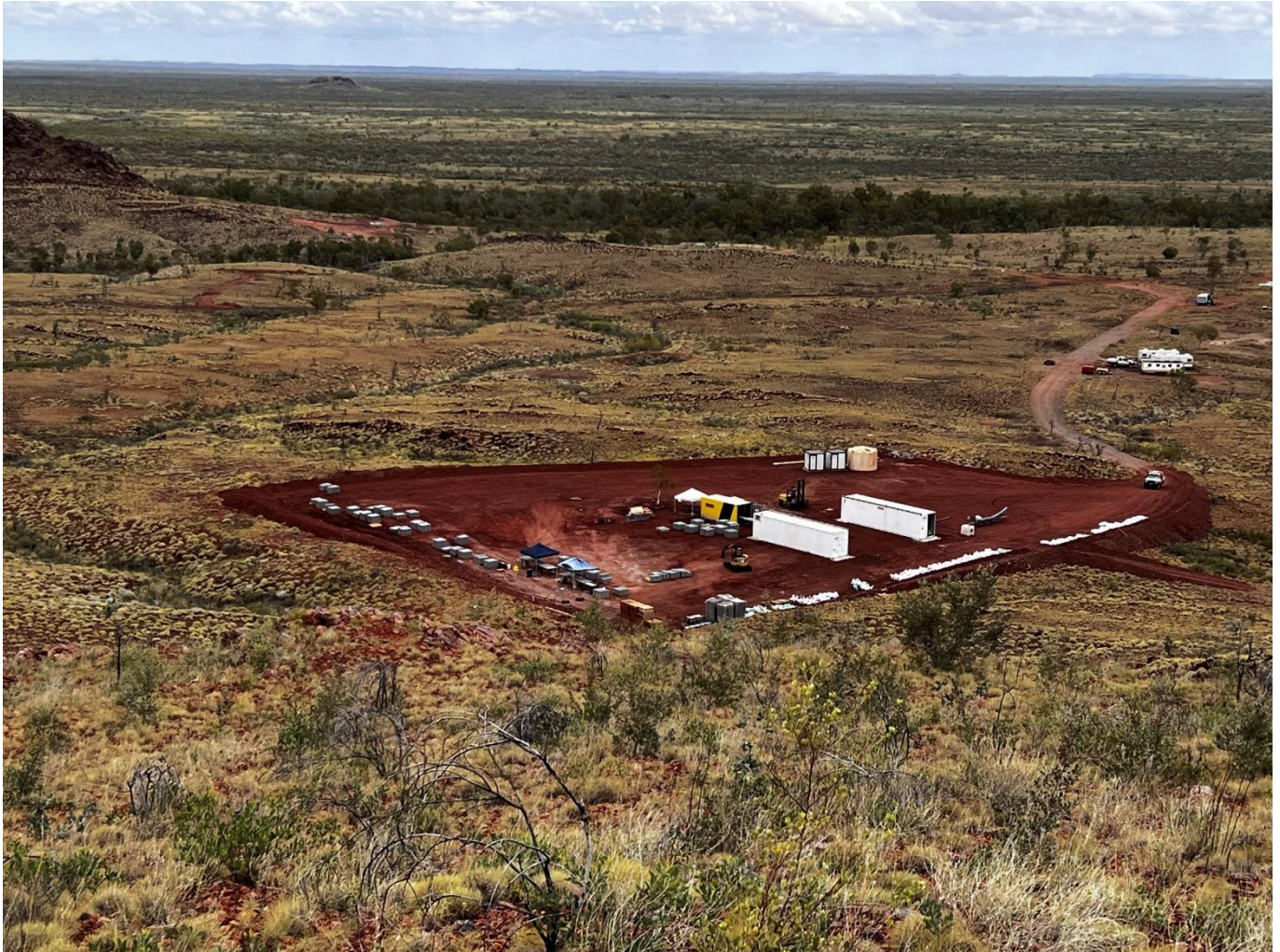
Figure 16 - Exploration camp construction underway with levelling and compaction of 70m x 70m area in preparation for dome-sheltered core yard, accommodation, ablution block, workshop and offices. The prominent hill in the background is the western part of the Main Hill deposit. View looking southwest.
